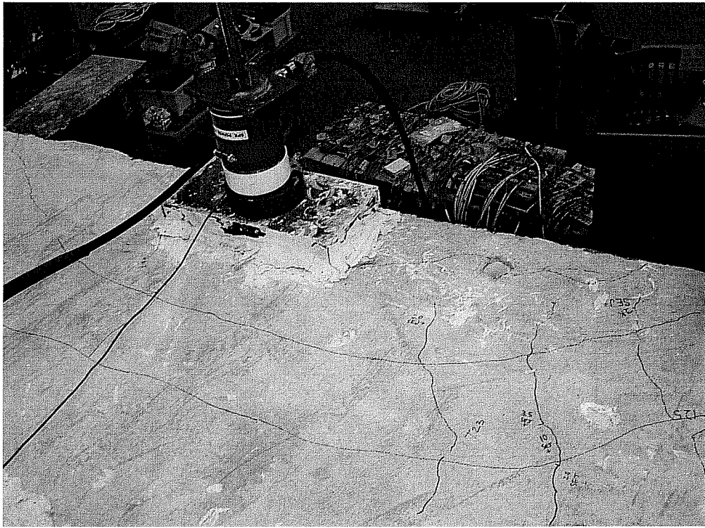
Figure 5.63 West exterior 10-ft bay failure at top of slab, facing northwest
