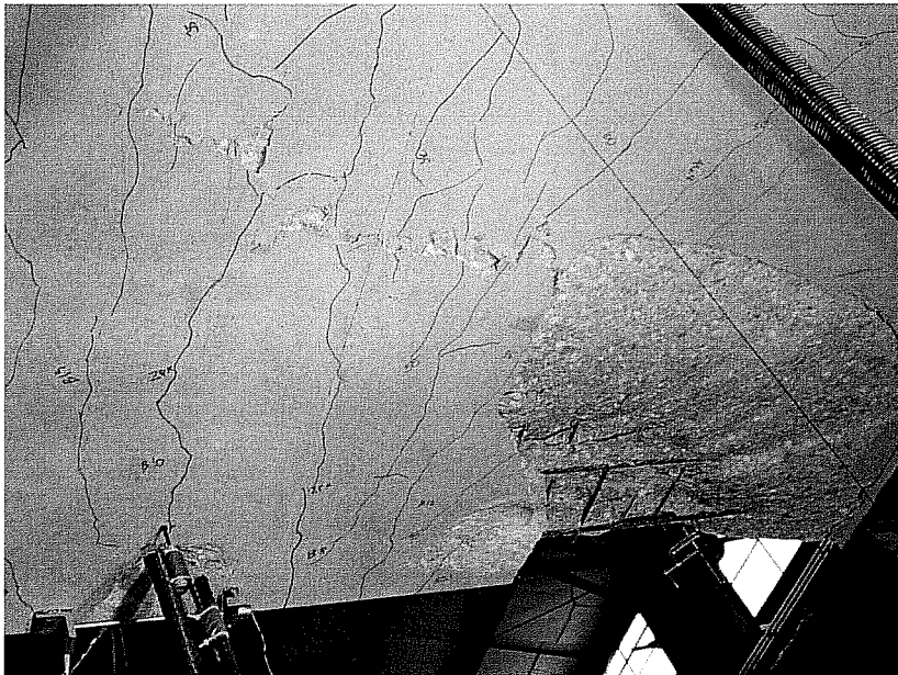
Figure 5.64 West exterior 10-ft bay failure at bottom of slab, facing northwest
