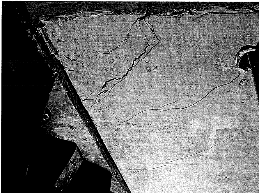
Figure 6.25 Failure of Overhang Test Area 3, bottom view, facing southwest
