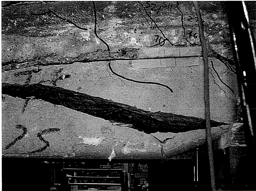
(b) Close up of delamination, facing north
