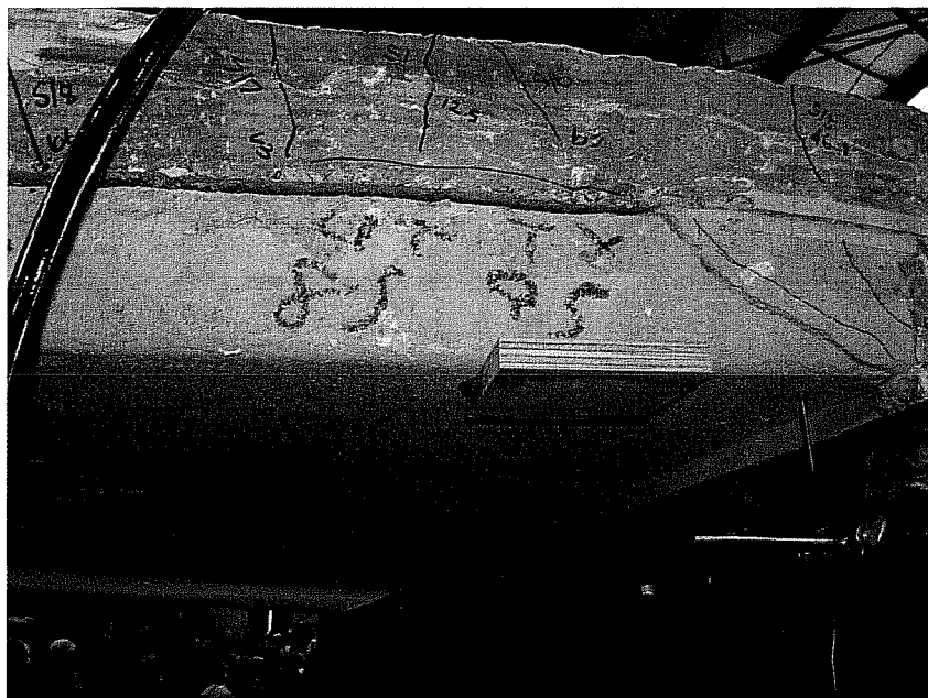
(b) Close up of delamination, facing north
